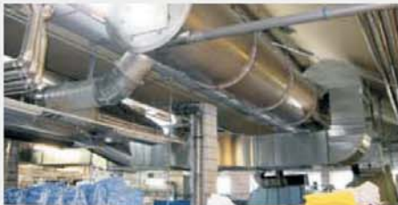
In the first expansion stage, the ceiling mounted exhaust air heat exchanger has already saved about EUR 8,000 per year.
