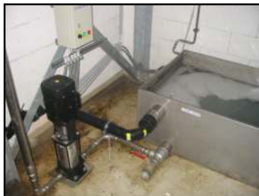
Photo: Spray water basin with spray water pump
