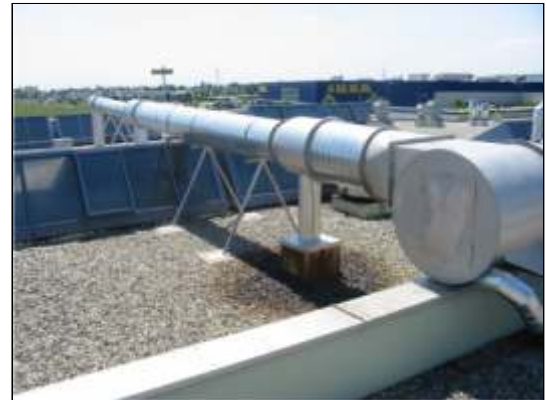
Photo: Example of exhaust piping into the spray tunnel
