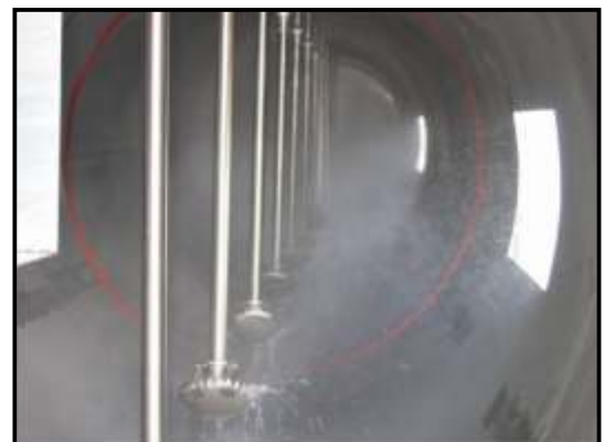
Photo: Spray water nozzles inside the spray tunnel create a water mist and purify the exhaust air
